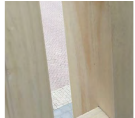
8.5 Reddish brown staining
